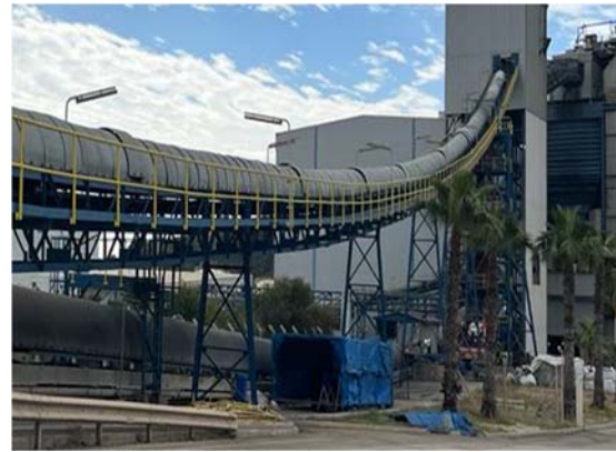
Figure 1. The conveyor line
